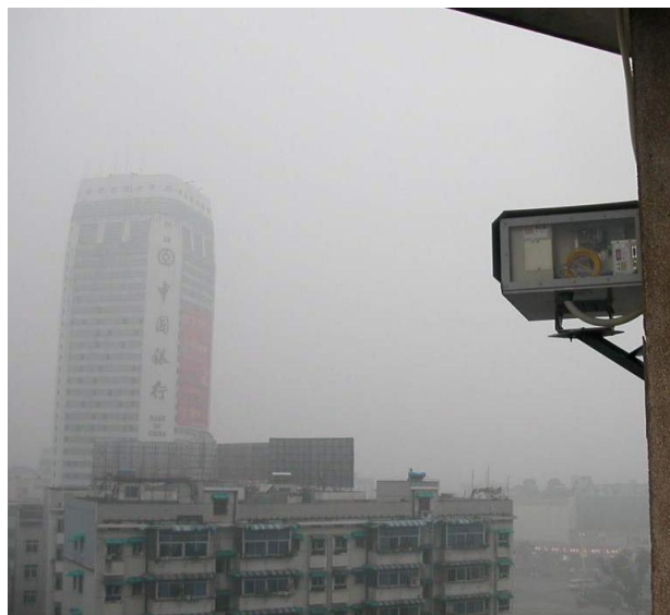
CableFree FSO deployed in Hunan Province, China. Industrial smog produces high attenuation which limits transmission distances to 1km. Sophisticated planning tools are used to predict link availability.
