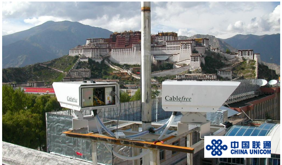
Last-mile application for China Unicom in Tibet. Shown here is a repeater site to provide non-line-of-sight connection from fibre ring to end-user site. Potala palace features in background.
